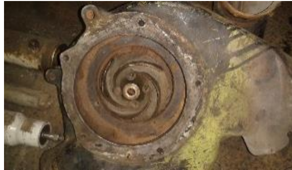
Figure 2: View from the pump's upper cover
